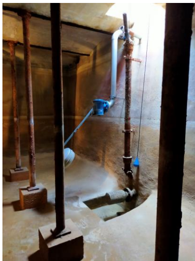
FIGURE 4 - PHOTO CANALISATIONS CORRODEES
