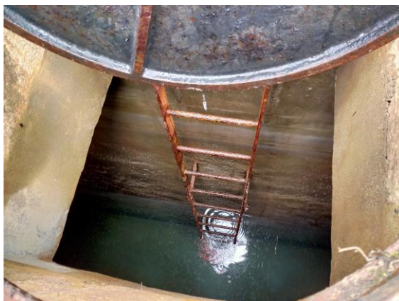
FIGURE 3 - PHOTO ECHELLE CORRODEE
